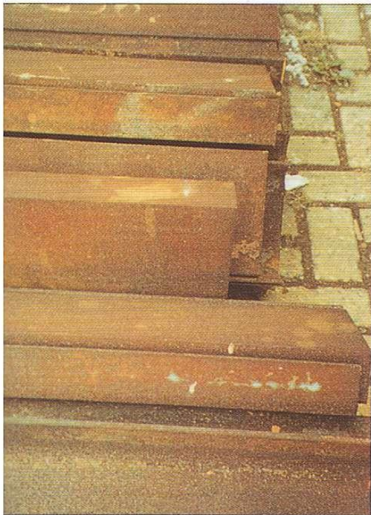
Channels. Surface condition clause: rusty
